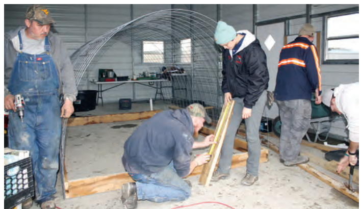
Refresh Appalachia farmer Wilburn Jude, left, supervises students Coby Gardener and Juli Vokes as they construct a chicken coop that will be used on the farm.
