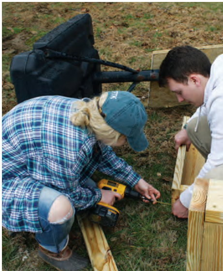
Building raised garden beds at Parkview Nursing and Rehab Center near Pikeville, Kentucky.
